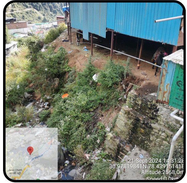
2. Dung and Waste water let out towards the river
